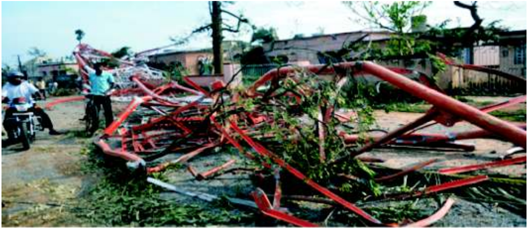
Mobile communication was totally disrupted: A damaged Mobile Tower
