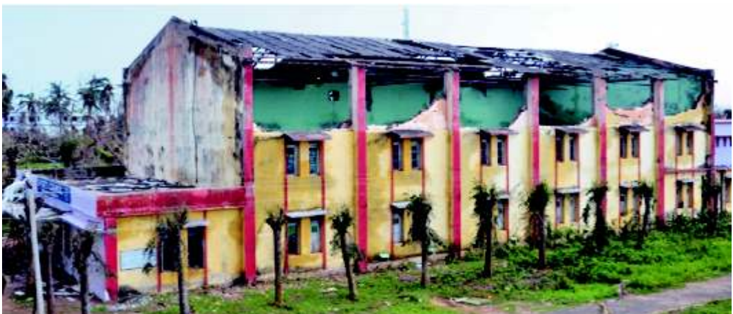
A damaged building in Berhampur University
