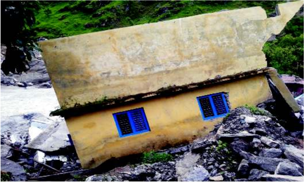
A house damaged due to deformed land beneath it.....
