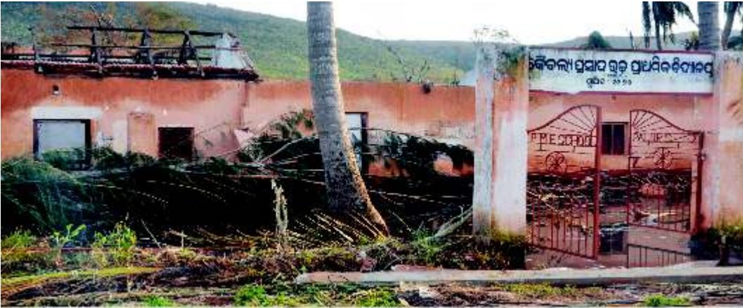
Damaged school building
