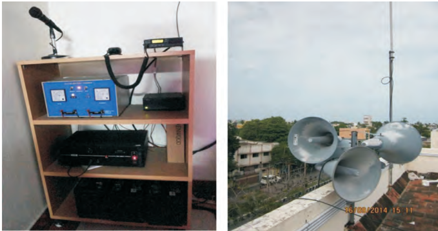
Photo 4: showing emergency operation centre.
