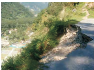
Damage to the edges of the roads
