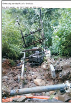
Damaged Electric Poles
