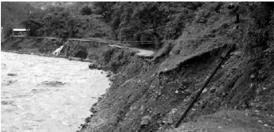
Fig 5: Damaged road near Uttarkashi (Source: DM Office, Uttarkashi).
