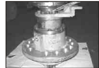
Fig 12 - (B) Bolt fouling at flange radius
